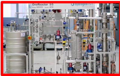
LOHC-System (300 kW / 150 MWh)
